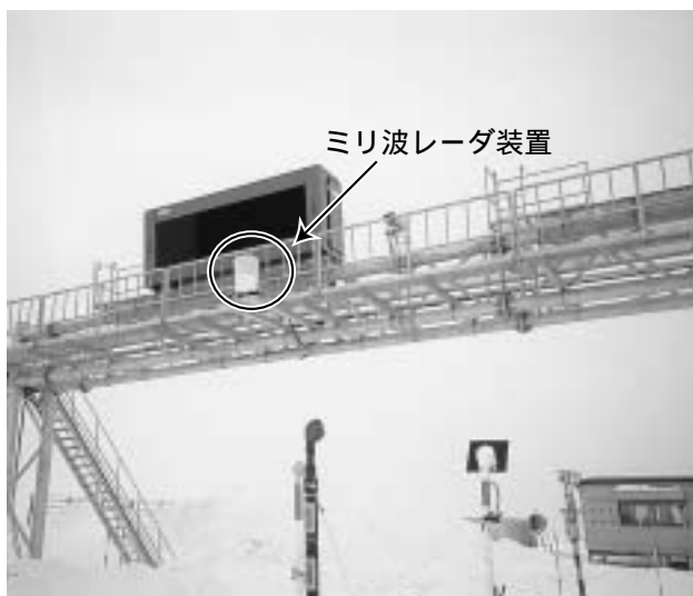
図-17 門構に取付けたミリ波レーダ装置 Fig.17 Millimeter-wave radar installed on the gantry
